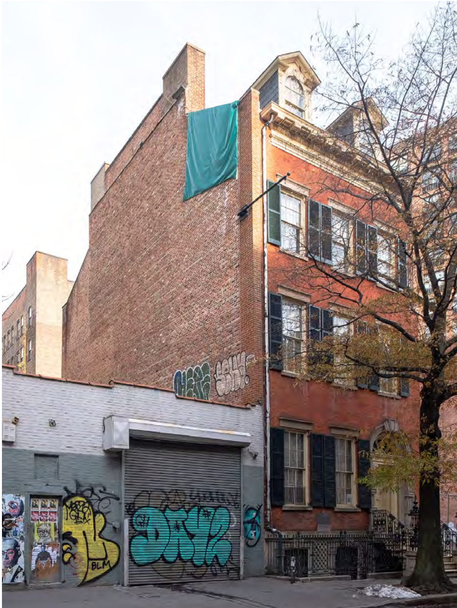
CURRENT LOT LINE WALL CONDITION
