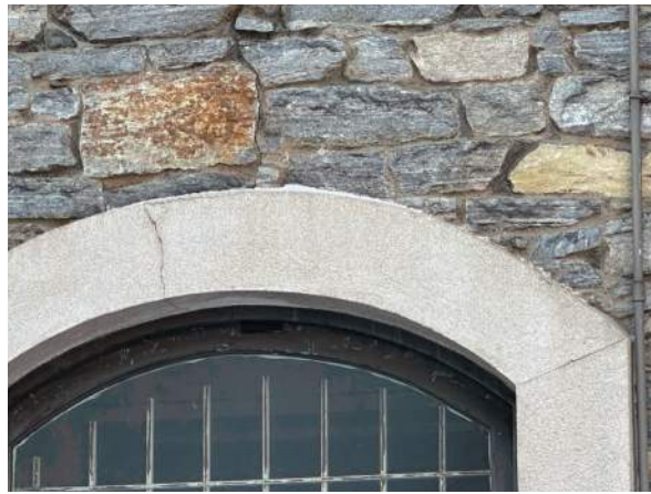
A11-1 - REPAIR CRACKS AT STONE MASONRY AND AT WINDOW SURROUNDS
