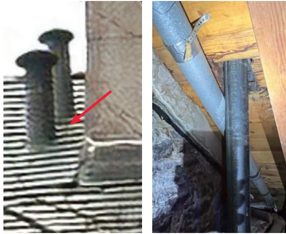
A02 - REPAIR FAILED ROOF VENT FLASHING
