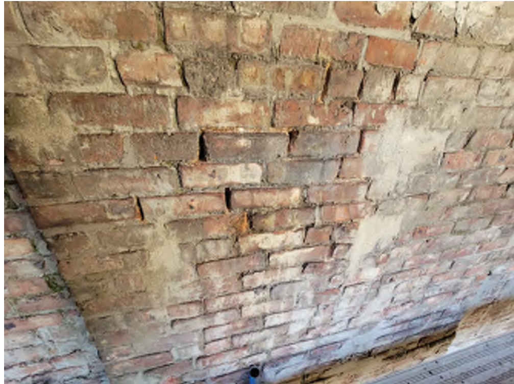
DEGRADATION OF FACADE BRICK (VISIBLE FROM SCAFFOLD)
