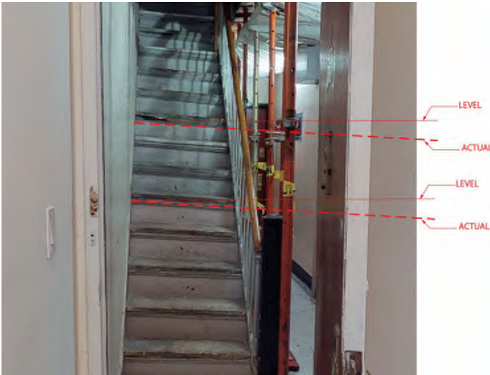
TILTED STAIRS DUE TO EXCESSIVE FLOOR JOIST DEFLECTIONS
