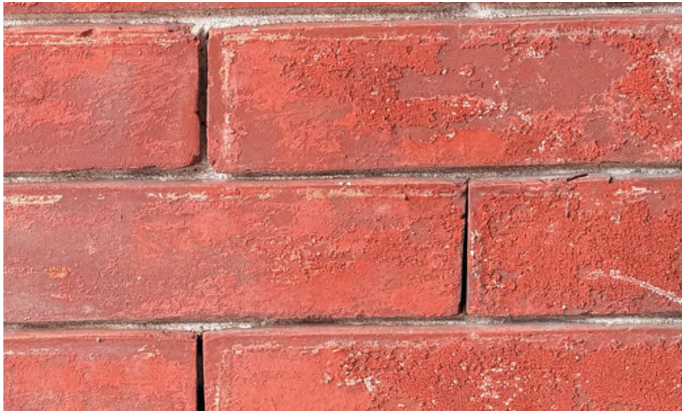
7 Former Coating Damage
