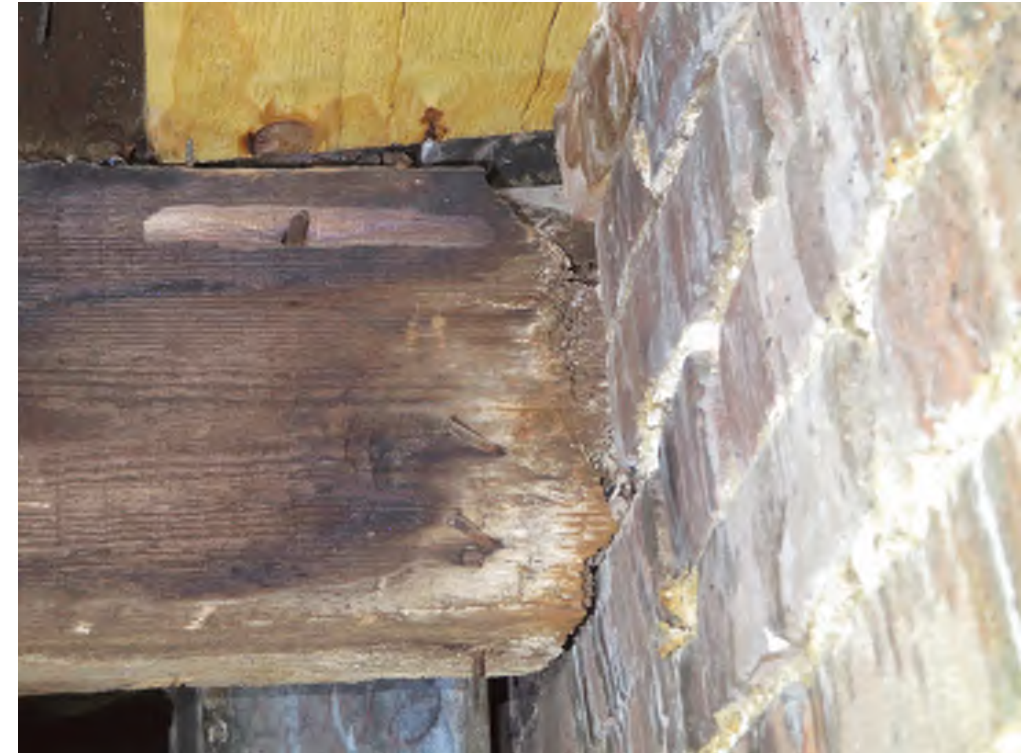
DEGRADED JOIST SLIPPING FROM POCKET
