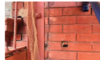
5. VERTICAL BRICK CRACK
