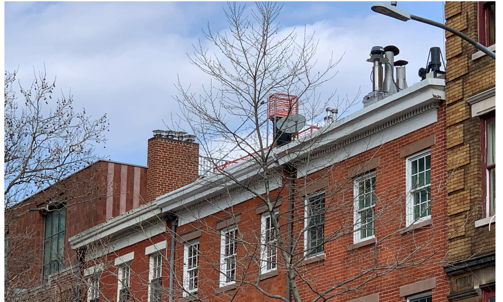
Detail view from west across Washington and Bank Streets, chimney extension is visible and penthouse fascia is minimally visible
