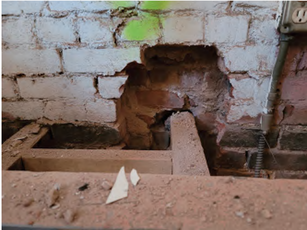
DEGRADED JOIST SLIPPING FROM POCKET
