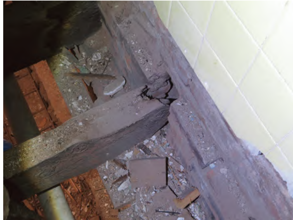
DEGRADED JOIST SLIPPING FROM POCKET
