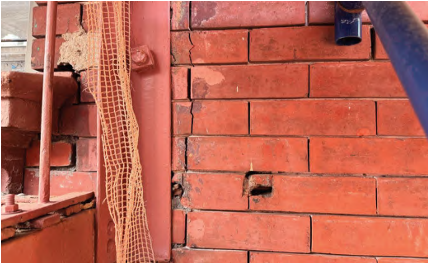
5 Vertical Brick Crack
