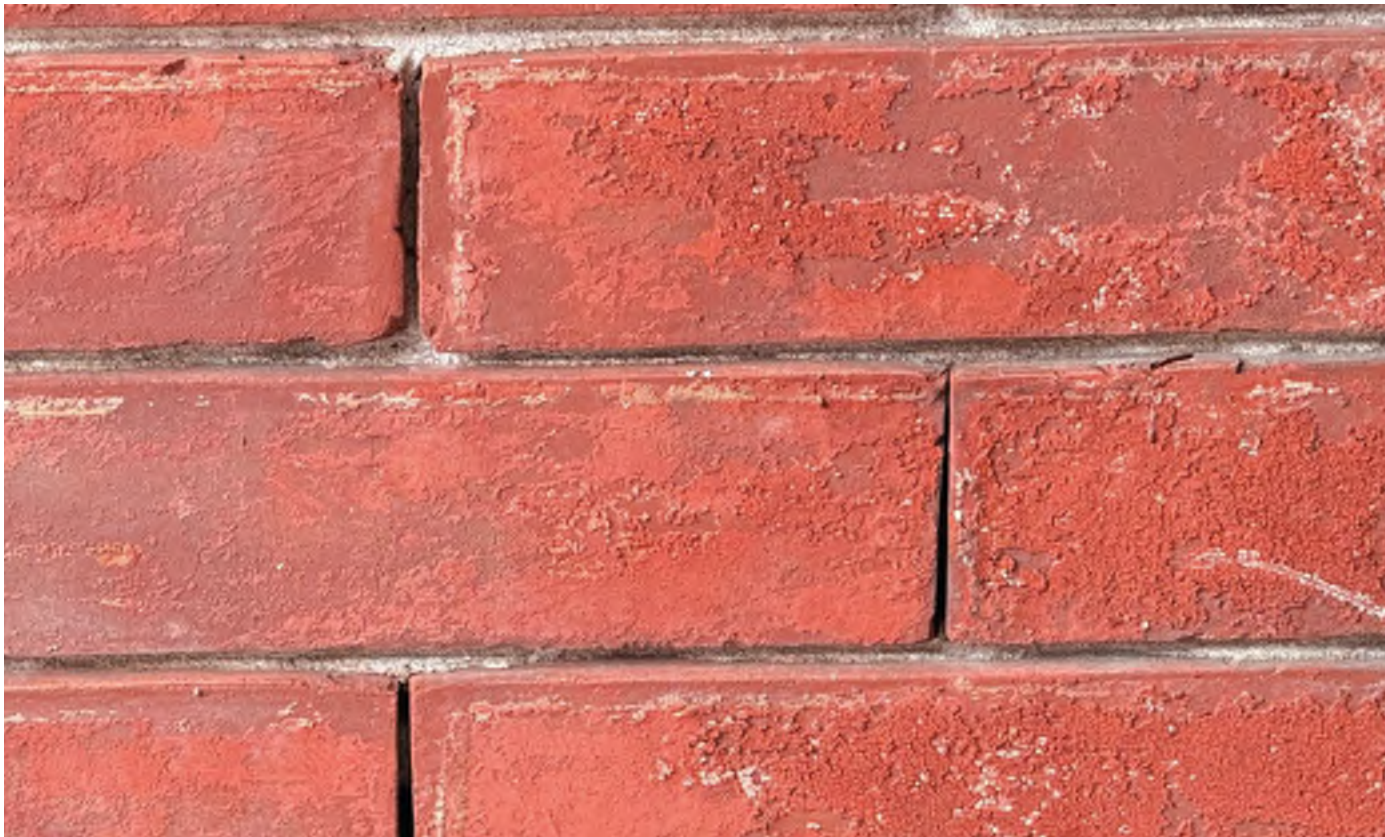
7 Former Coating Damage
