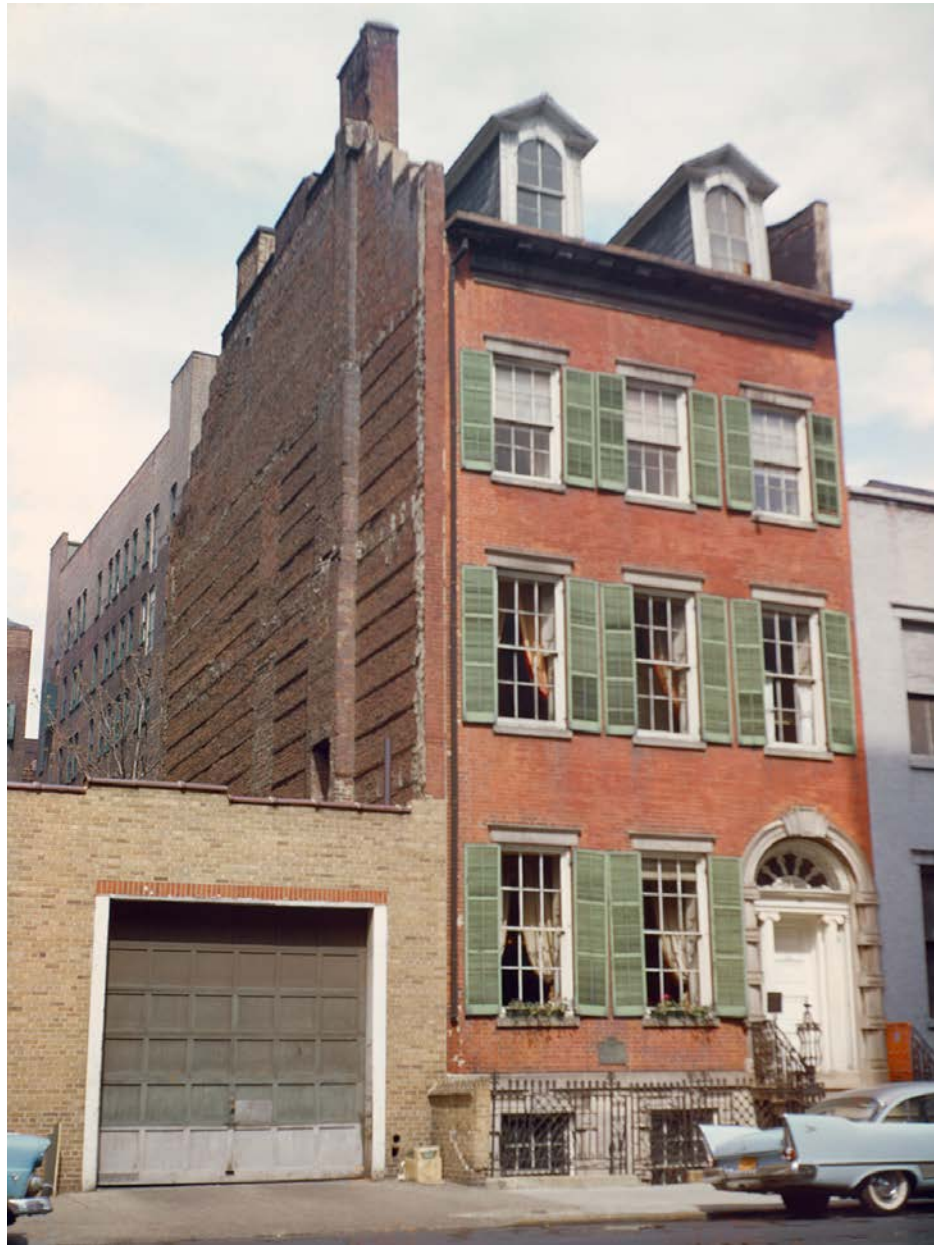
1960'S LOT LINE WALL CONDITION
