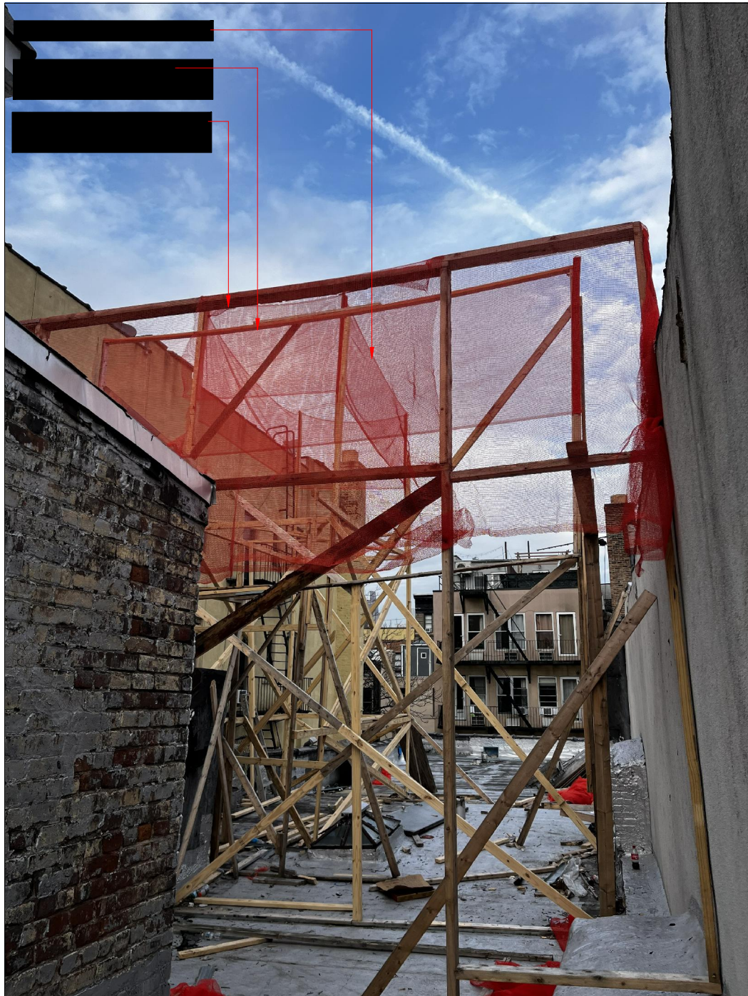
Street wall at 4th floor, mezzanine & stair bulkhead (view from west of tower)
