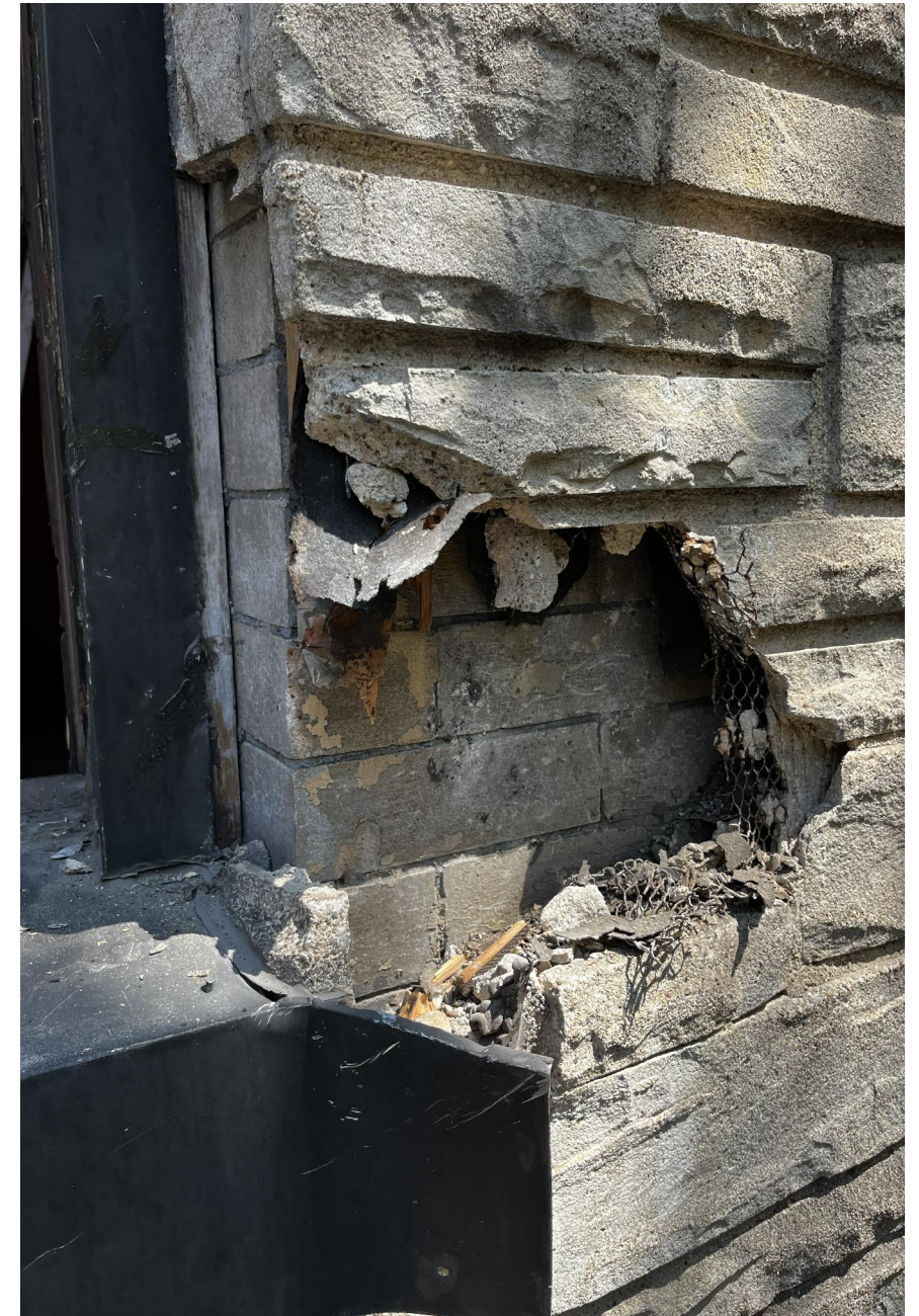
Probe at 2nd floor window - exposed brick under faux stone cladding
