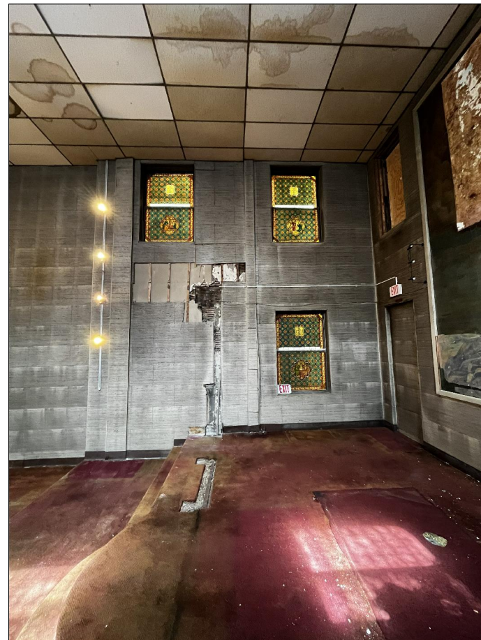
Faux stain glass film at sanctuary windows
