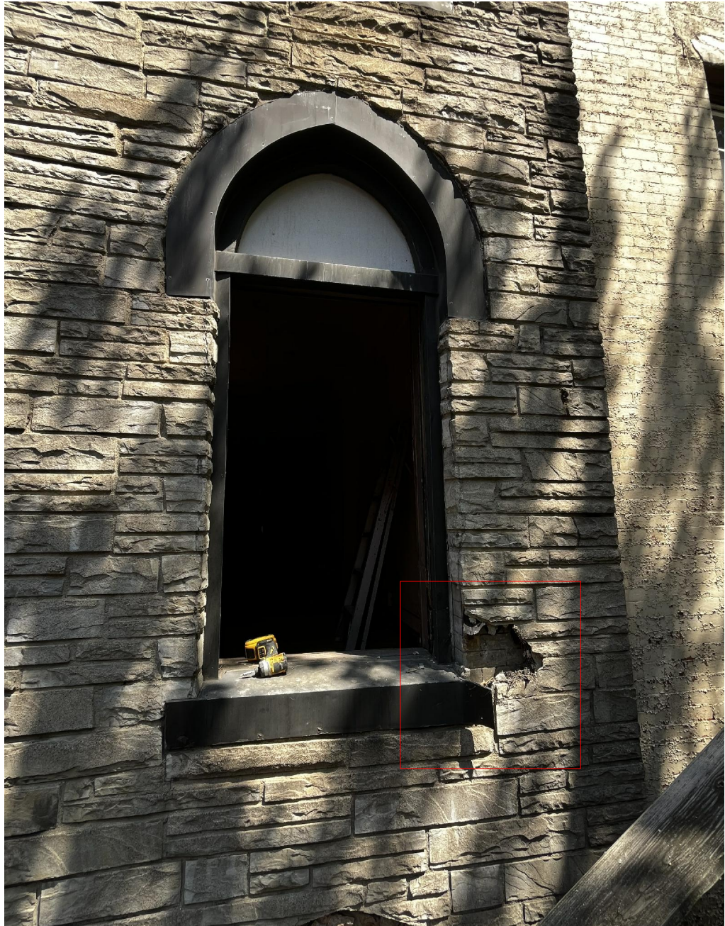
Exterior view at 2nd floor window - faux stone removed to reveal existing brick facade
