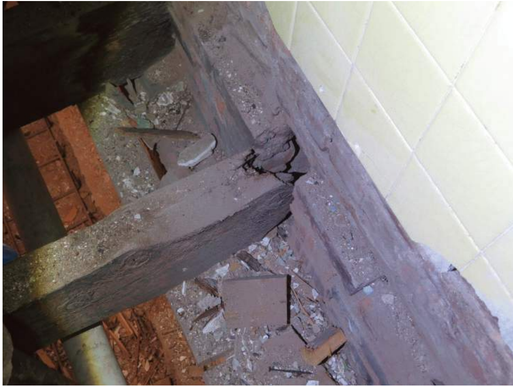
DEGRADED JOIST SLIPPING FROM POCKET
