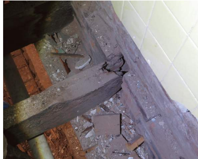
DEGRADED JOIST SLIPPING FROM POCKET
