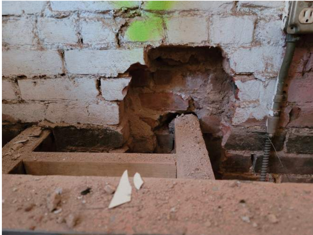
DEGRADED JOIST SLIPPING FROM POCKET
