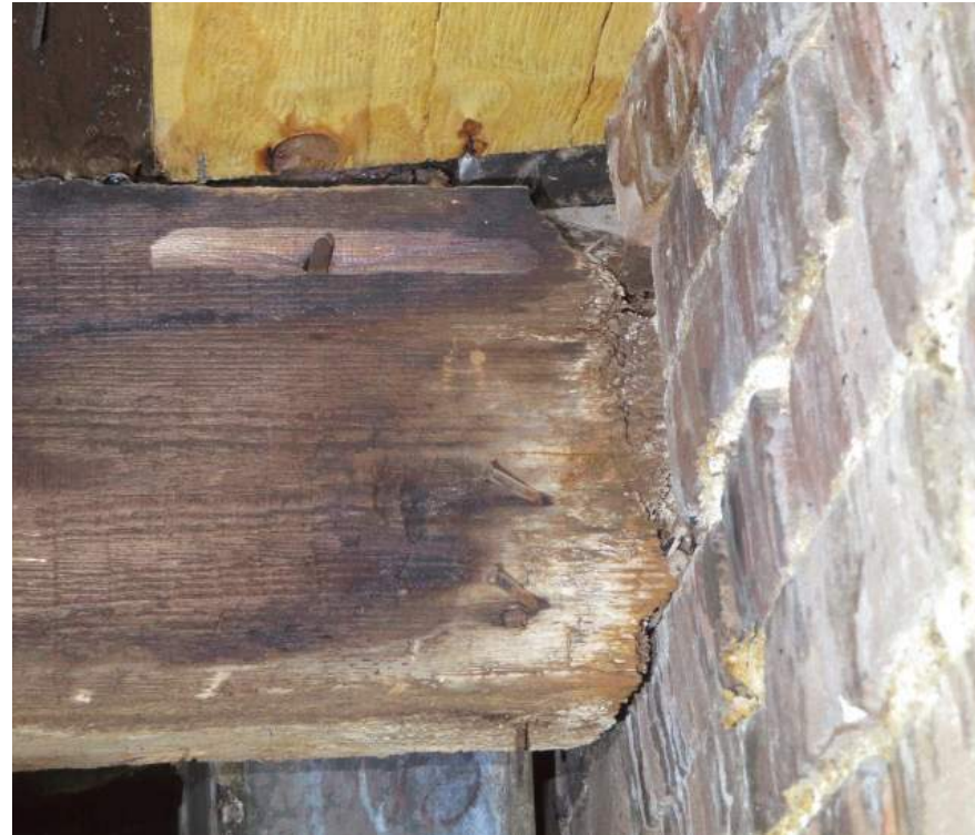
DEGRADED JOIST SLIPPING FROM POCKET
