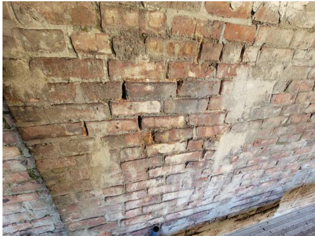
DEGRADATION OF FACADE BRICK (VISIBLE FROM SCAFFOLD)
