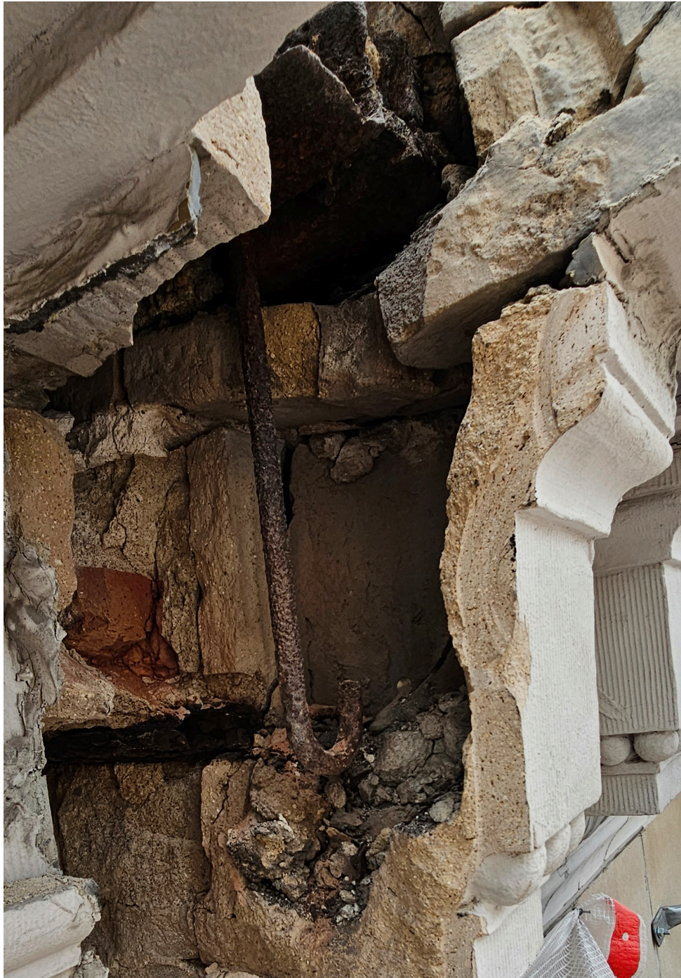
Deterioration of steel anchor embedments
