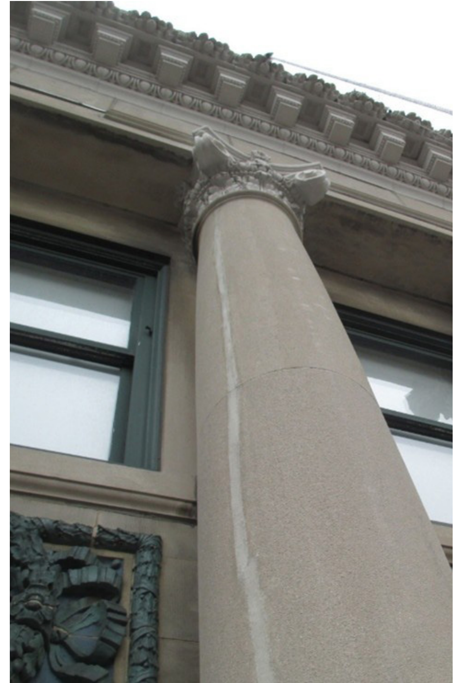
Continuous vertical cracking at limestone due to compression forces
