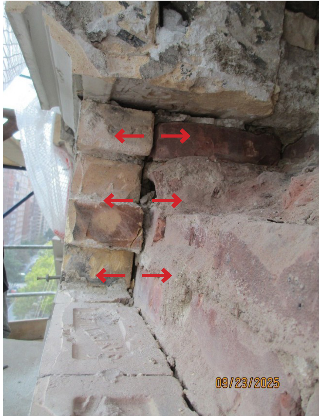
Separation between face brick and back-up brick masonry back up wall due to lack of header course
