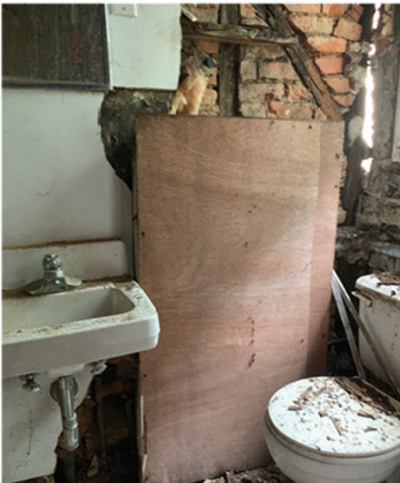
Interior deterioration due to weather infiltration at open exterior corner
