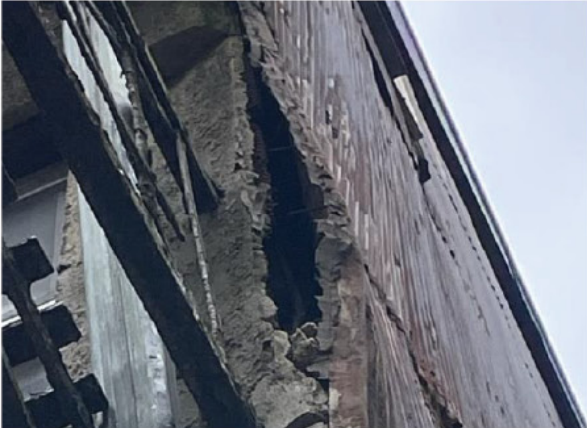
Buckling Wall Separation of the north and east wall, source of considerable water infiltration
