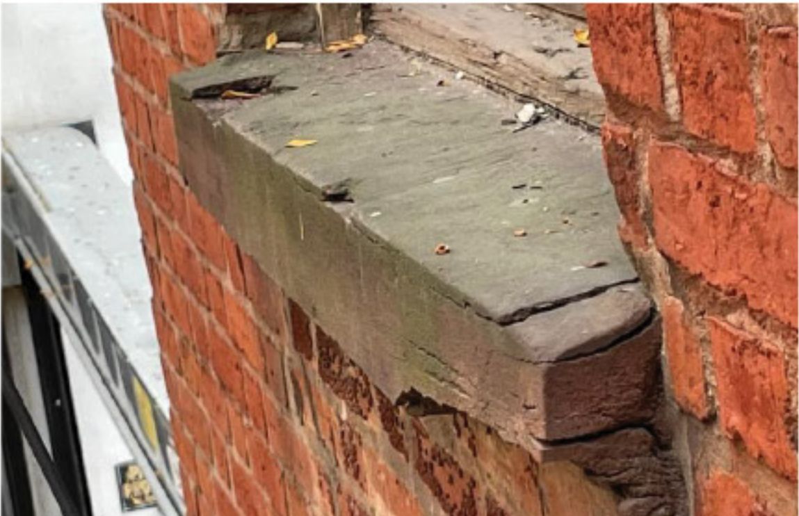
Stone Sill Deterioration
