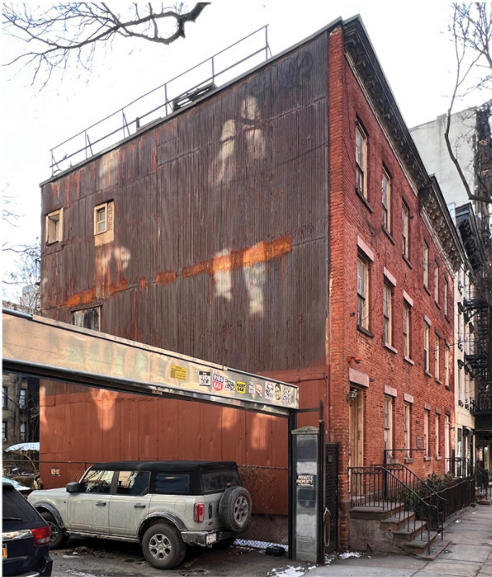
85 Sullivan Street North Facade Current photograph, deteriorated metal cladding, installed in 1930s
