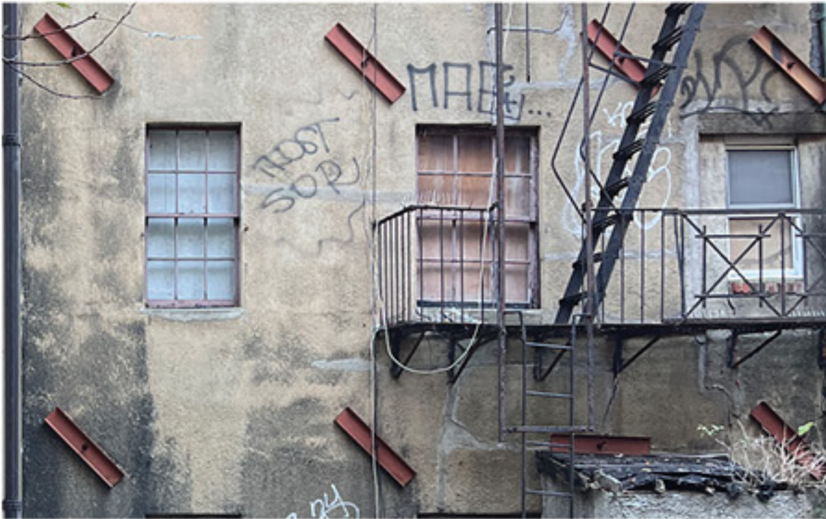
Exposed Structural Tie-Backs Installed in 2009 to help stabilize the building and prevent further separation of the facade
