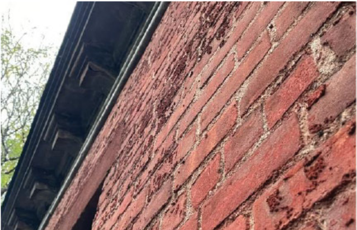
Flaking Paint Residue
