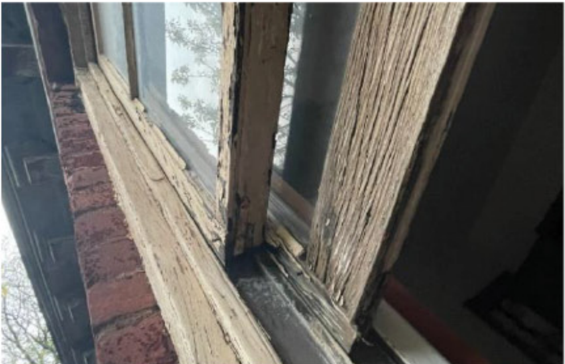
Severe Window Frame Deterioration
