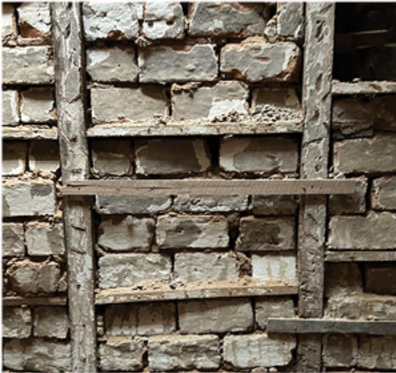
Decay of brick nogging wall, including loose brick and rot at original structural timbers
