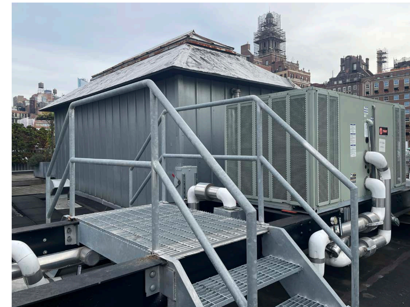
6. EXISTING HVAC EQUIPMENT
