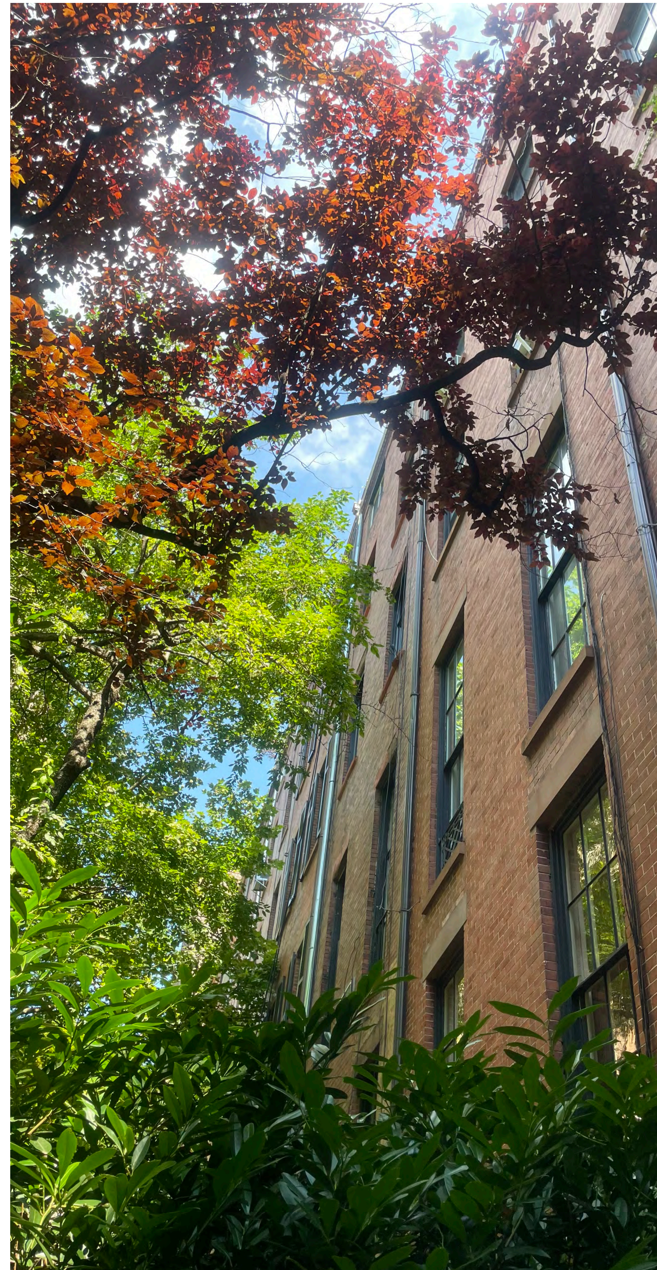
2A. NEIGHBORS FACADE EXTENSIONS AS VIEWED FROM 24 W 10TH ST BACK YARD (JULY 2025)
