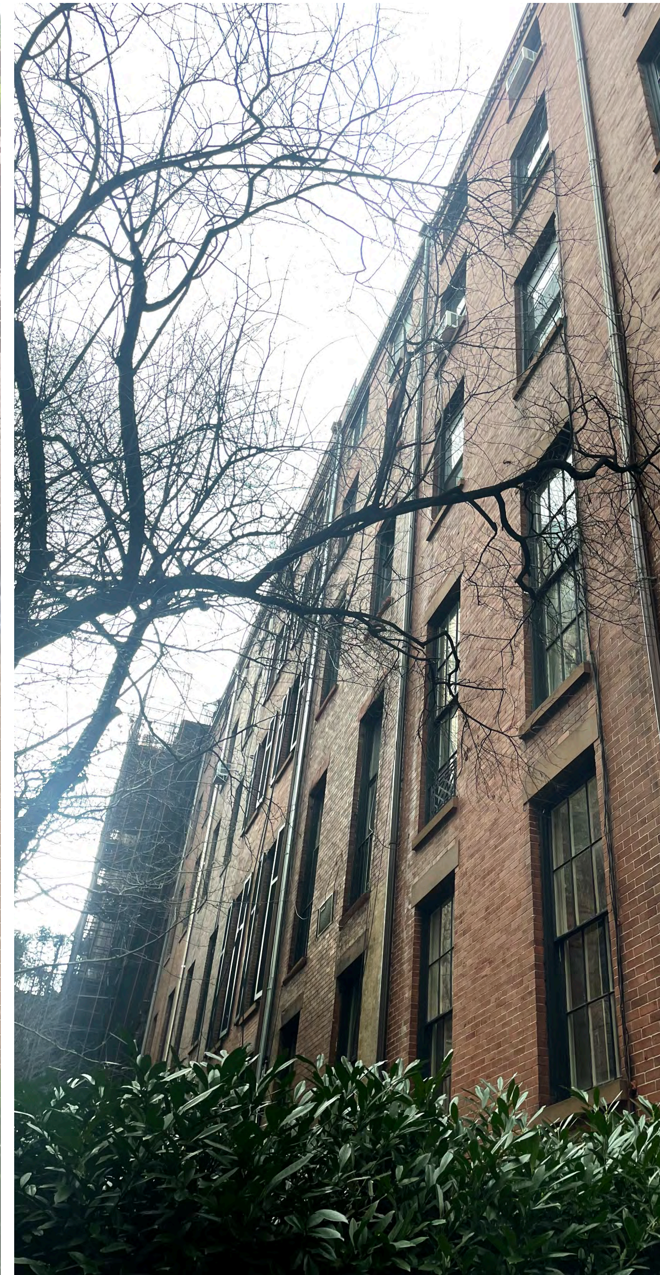
2B. NEIGHBORS FACADE EXTENSIONS AS VIEWED FROM 24 W 10TH ST BACK YARD (JAN 2025)
