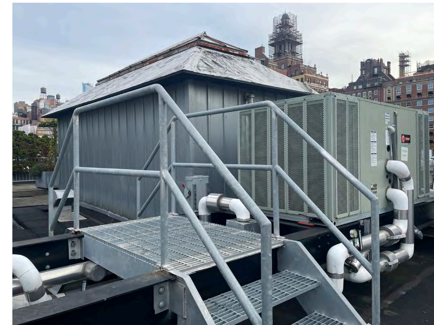
6. EXISTING HVAC EQUIPMENT
