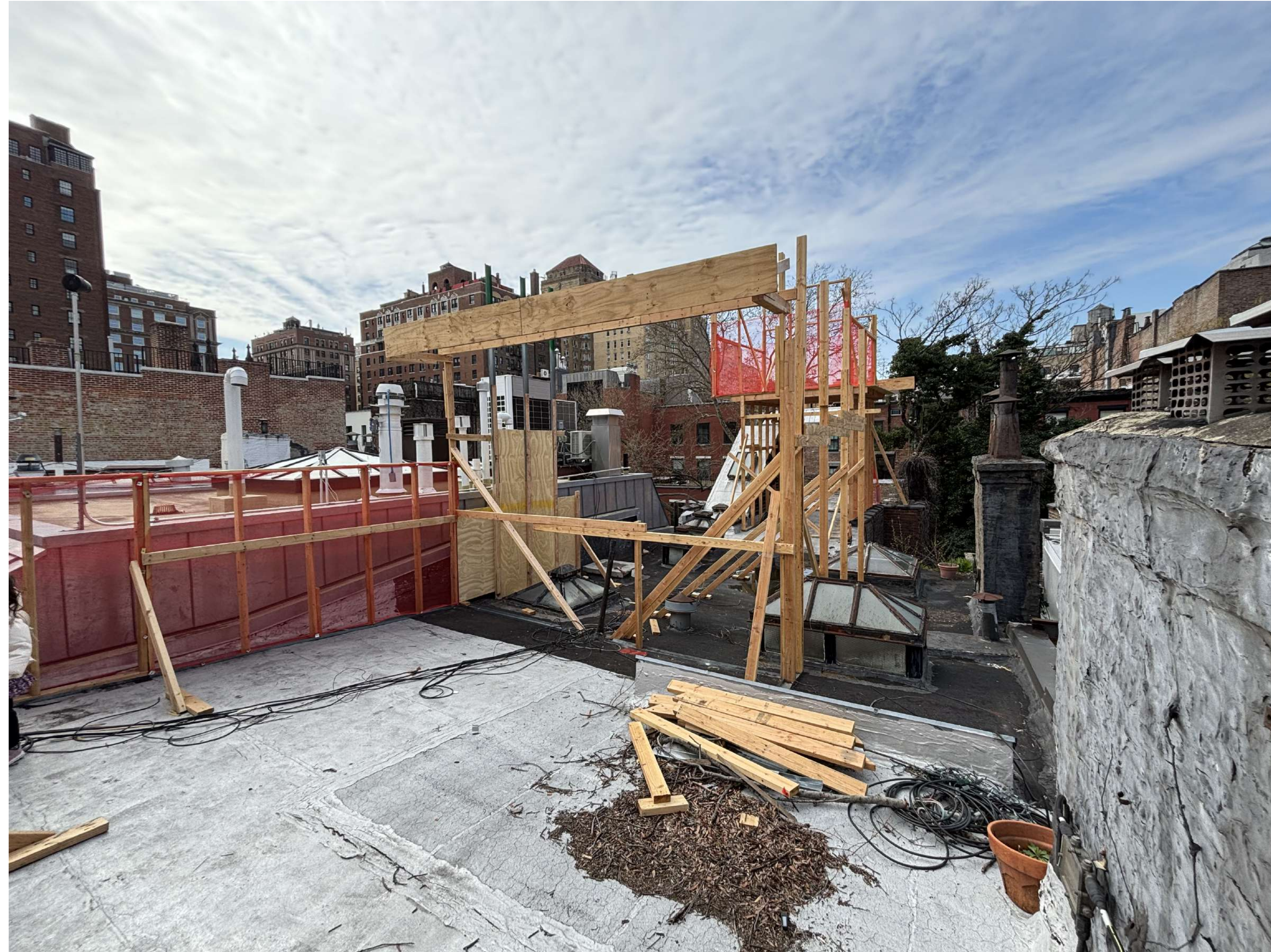
VIEW OF 4TH FLOOR PENTHOUSE & MECHANICAL SCREEN MOCKUP LOOKING TOWARDS REAR YARD
