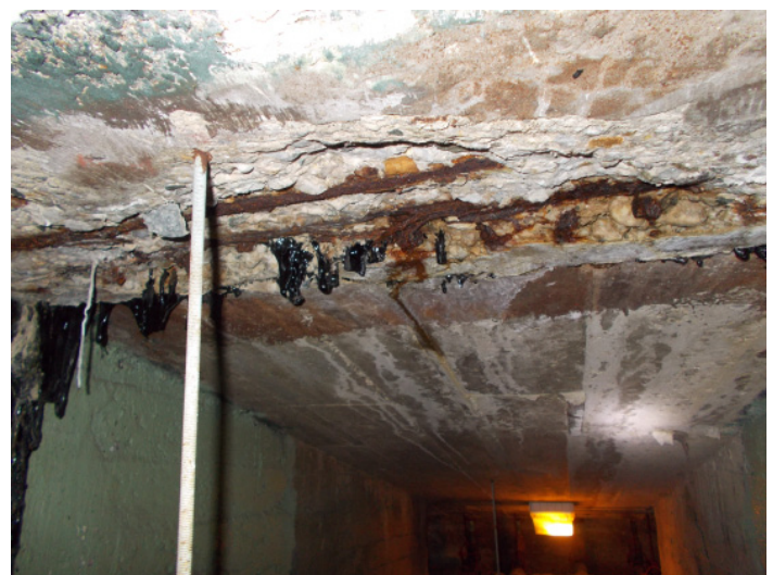
Leaks in Pool Shell
