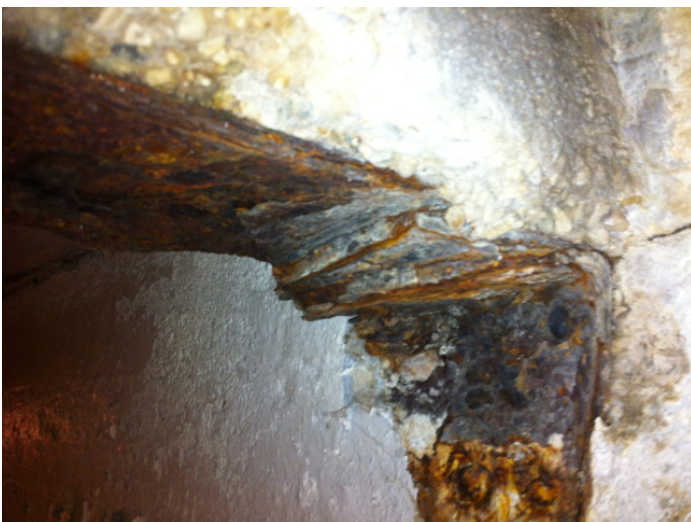
Deteriorated Structure at Sidewalk Vaults
