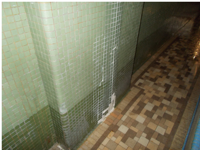
Pool Finishes Exhibiting Moisture Damage
