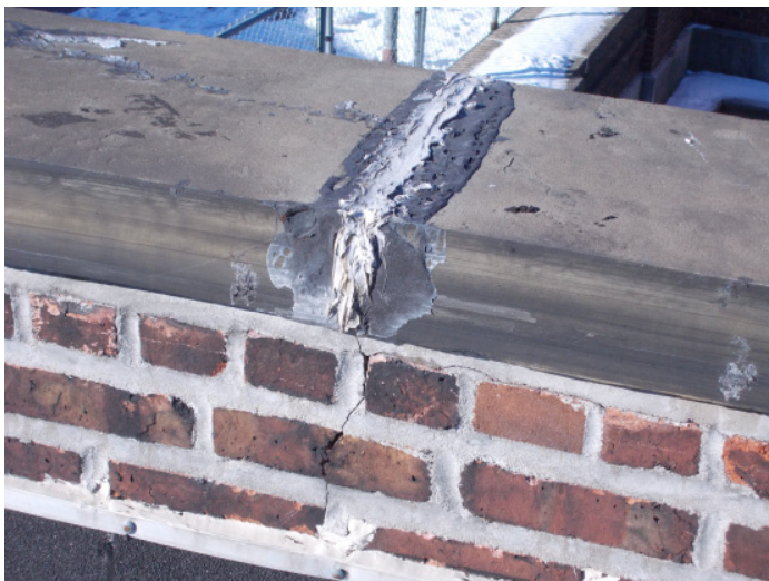
Parapet and Coping Deteriorated Joints
