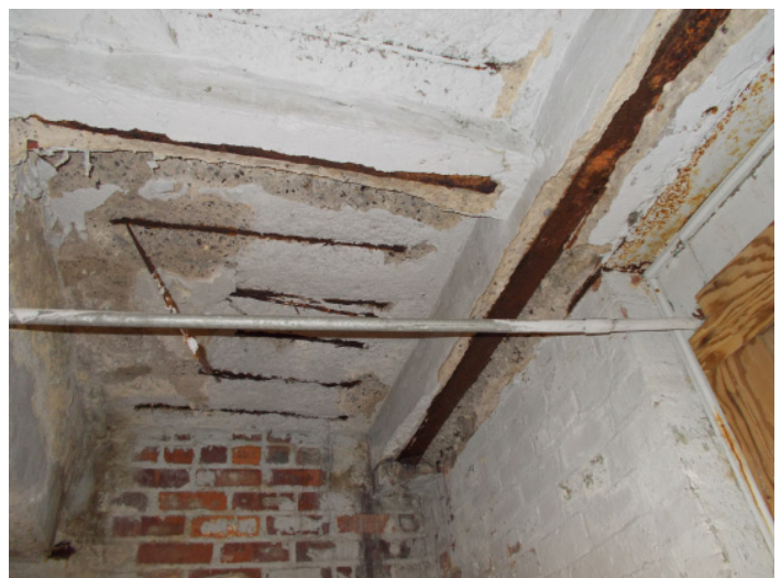
Basement Level Exposed Rebar
