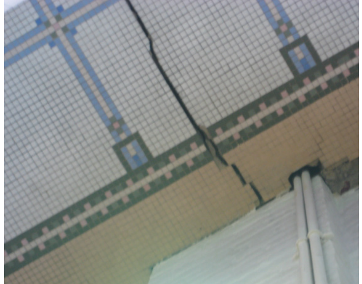
Gym Ceiling Expansion Crack in Tile Finish
