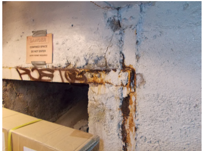
Abandoned Coal Chute with Deteriorated Lintel
