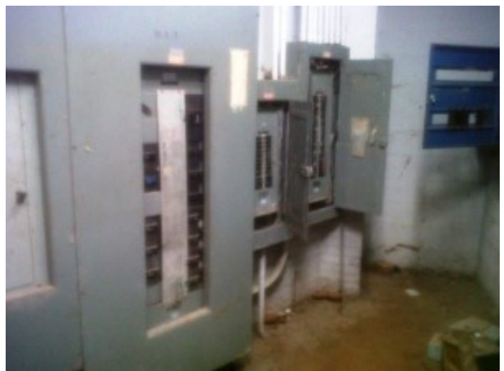
Electrical Room - Flooded During Hurricane Sandy
