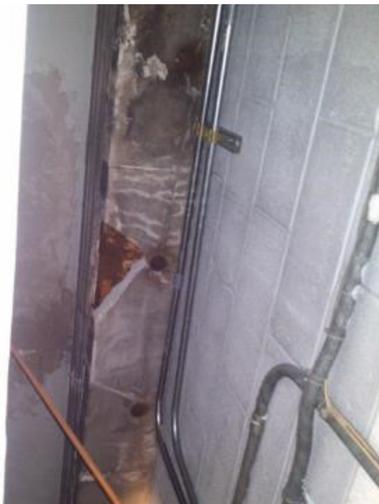
Falling Limestone at 3rd Floor Mechanical Room
