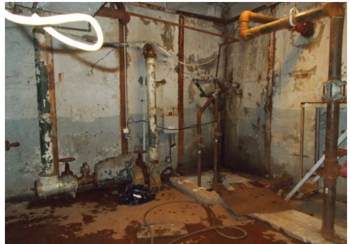
Priority 2 - Sidewalk Vault - Deteriorated Structure
