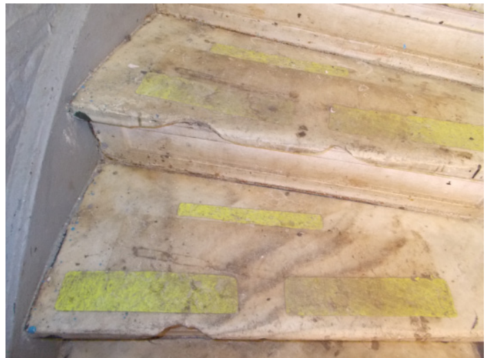
Winder Stair with Broken Treads
