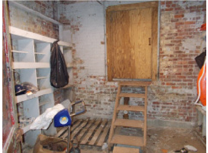
Basement Level Plywood Door at Second Means of Egress
