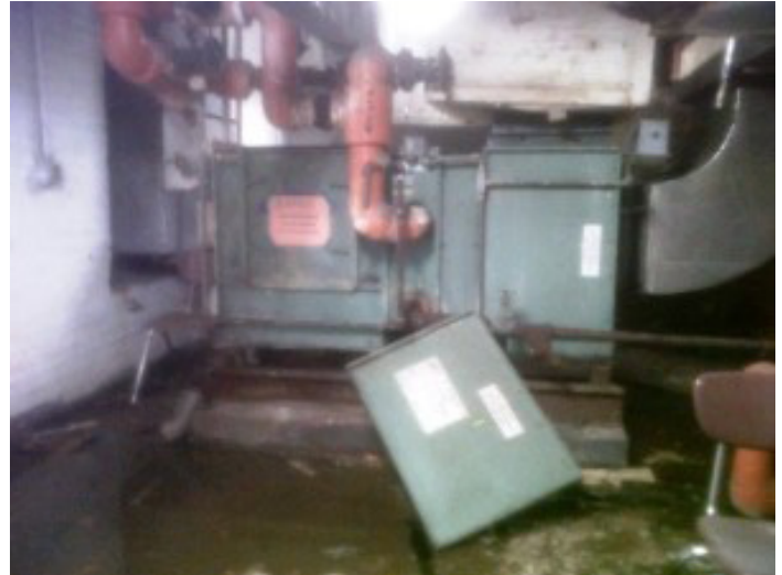
Air Handler Serving Locker Rooms
