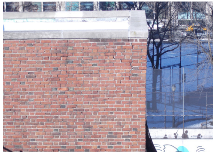
Priority 1 -Stair 3 Tower with Separating & Canting parapet
