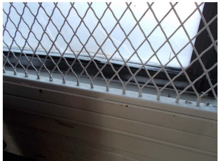
Damaged Window due to Masonry Settlement
