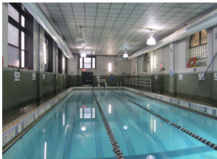
Indoor Pool - Non-Code Compliant Narrow Deck
