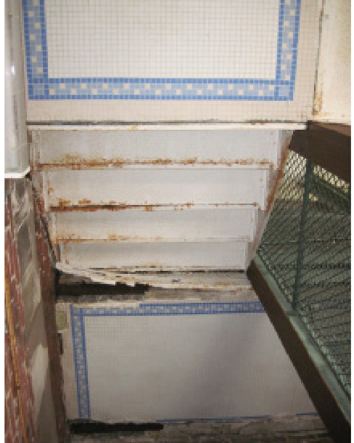
Priority 1 -Stair 3 Tower with Corroded Structure and finishes
