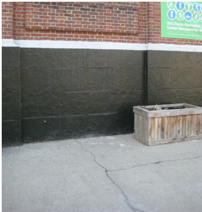
Priority 2 - Sidewalk Cracking above Deteriorated Vault Structure
