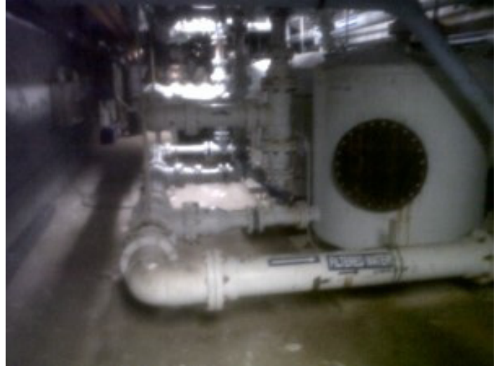
Pool Filter Room Steam Piping
