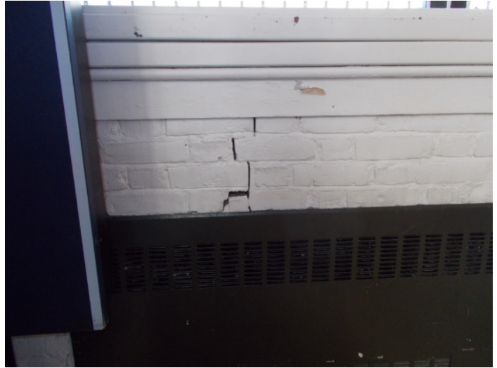
Priority 2 - Masonry Settlement Causing Window Cracking
