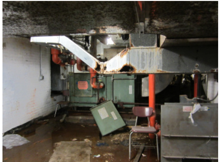
Antiquated and Deteriorated Mechanical Systems
