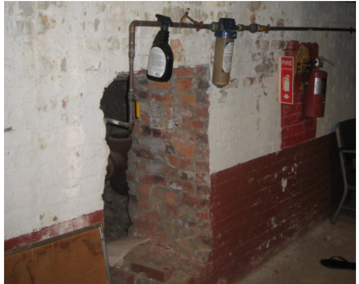
Unsupported Opening in Bearing Foundation Wall
