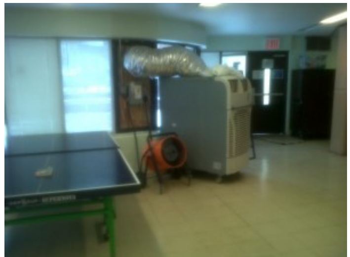
3rd Floor Temporary AC in Multi-Purpose Room
