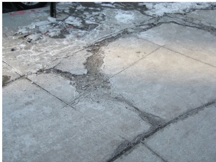
Spalls in Public Sidewalk
