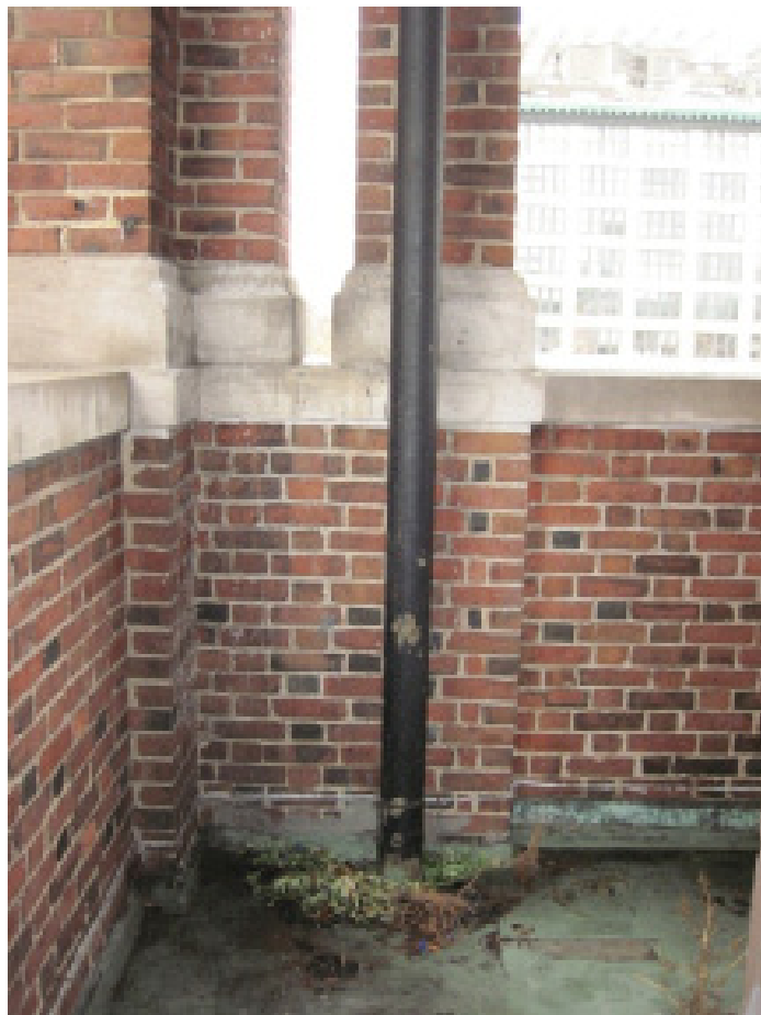
Deteriorated Roof Leader at Colonnade Loggia w/ plant growth
