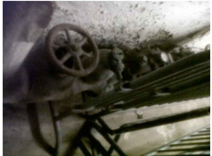
Domestic Water from Sump Pump Room
