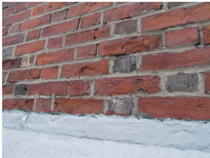
Spalling Brick due to Inappropriate Repointing Mortar
