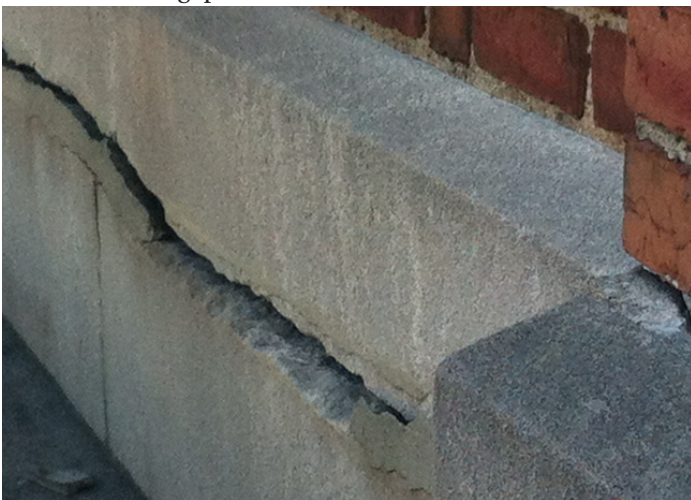
Rooftop Colonnade / Loggia - Cracks at Limestone Band
