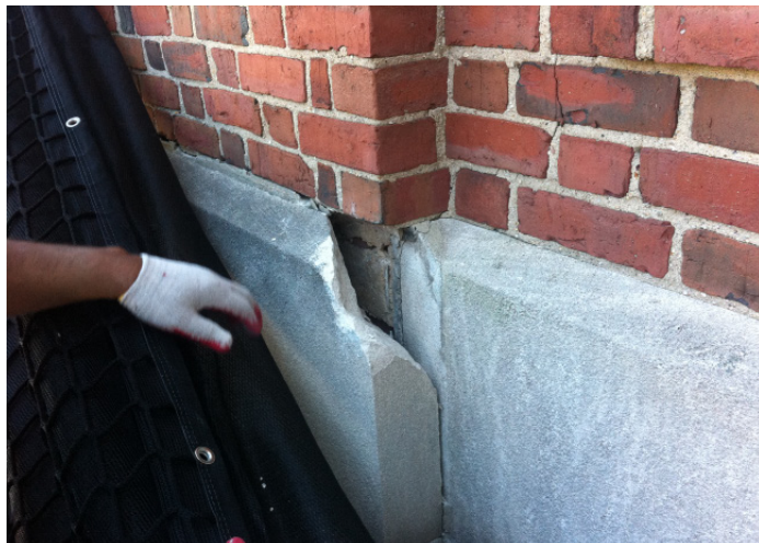
Priority 1 -Colonnade Loggia cracked and Spalled Limestone
