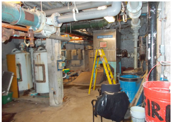
Priority 2 - Replacement of Antiquated MEP
