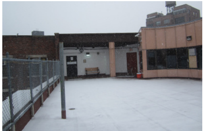
Computer Room Access across Roof
