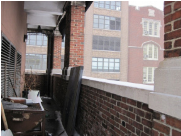
Priority 1 -Colonnade Loggia with Spalling Stucco & Open Joints
