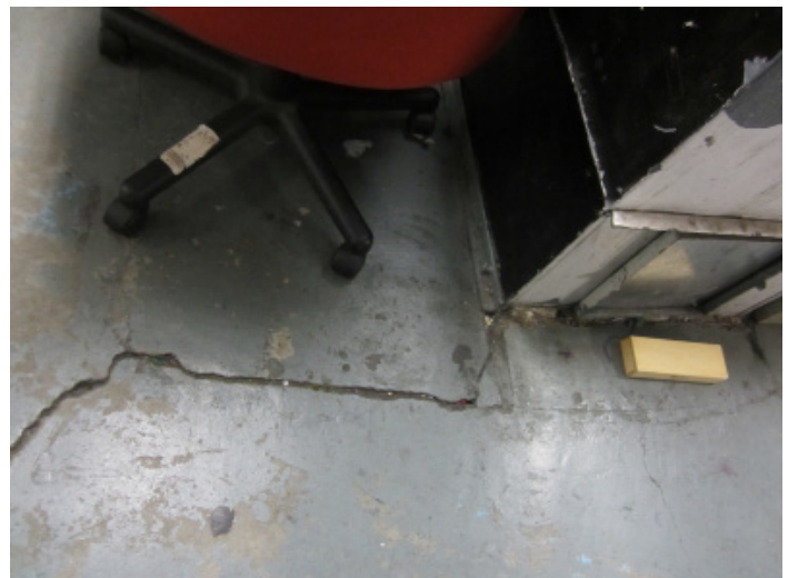
Crack in Floor of Third Floor Mechanical Room
