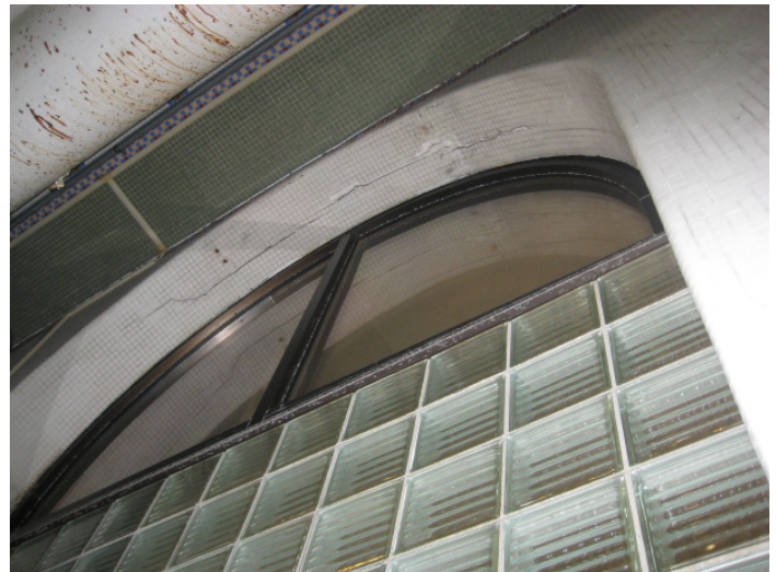
Pool - Cracks at Window Arch
