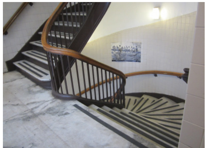
Primary Egress Stair - Non-Code Compliant Winder Stairs
