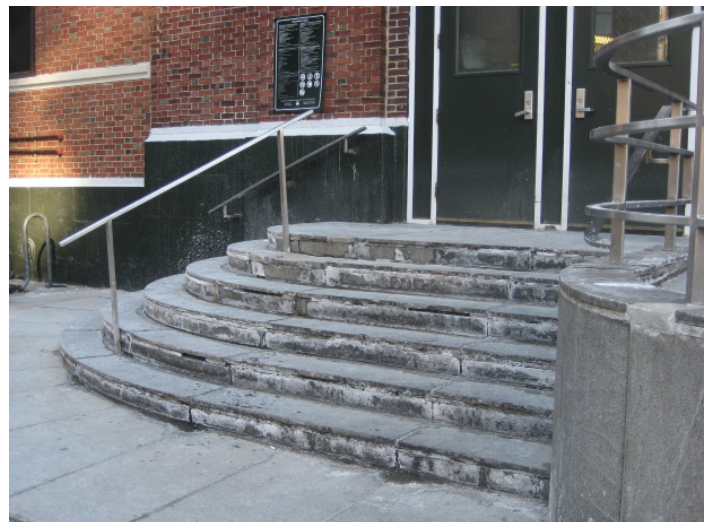
Entrance Stair / Ramp - Open Joints Allowing Water Infiltration
