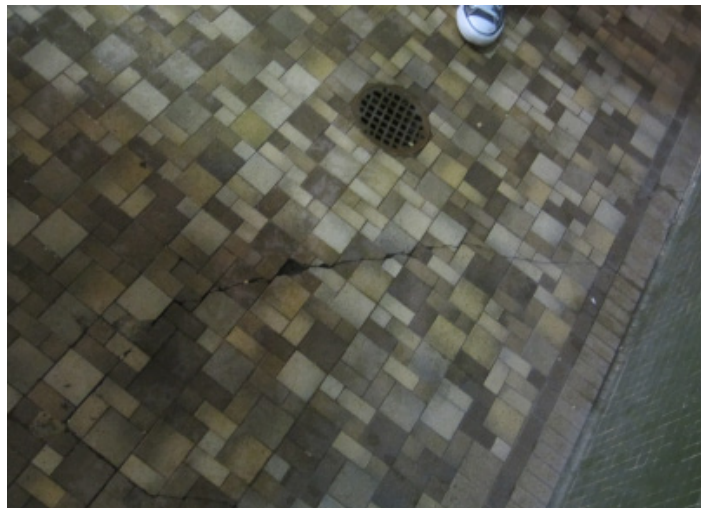
Indoor Pool - Crack in Deck by Drain
