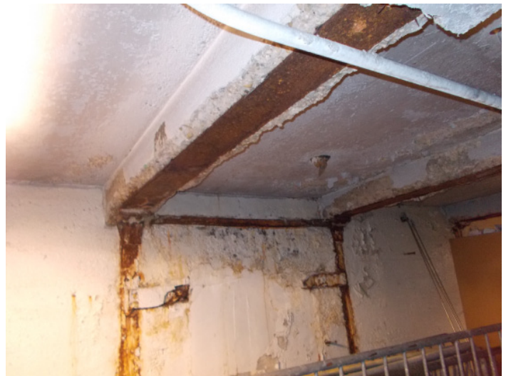
Sidewalk Vault Deteriorated Structure
