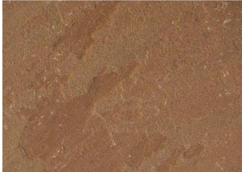
(EXISTING) BROWNSTONE EXTERIOR STONE; MATCHING BROWNSTONE STUCCO TO BE USED FOR PATCHING LOCATIONS; BROWNSTONE-STYLE CAST STONE TO BE USED FOR LINTELS AND SILLS
