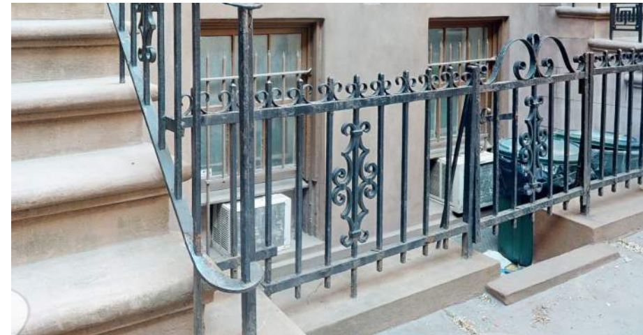
CURRENT 180 WAVERLY RAILING TO BE REPLACED
