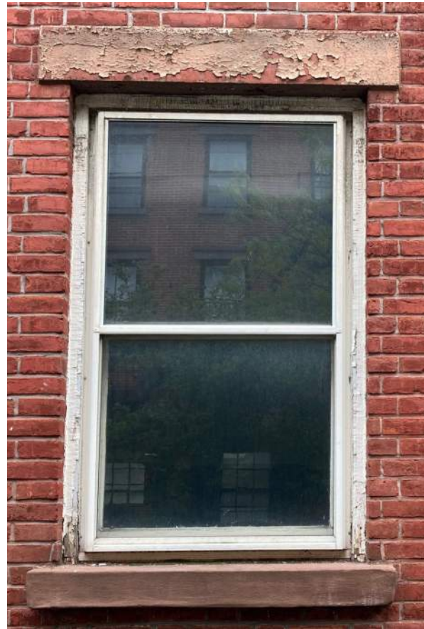
front and rear existing windows replace existing to match (white finish) Restore existing window sills and headers
