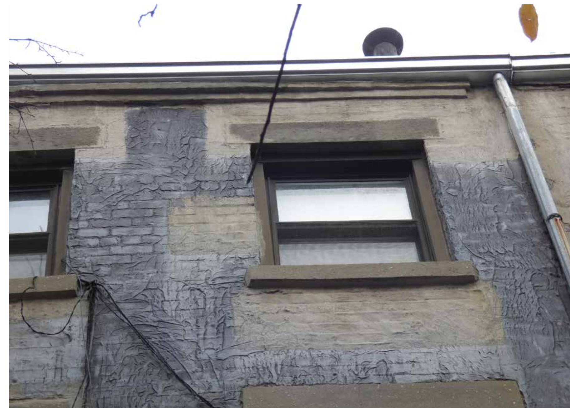
TOP FLOOR WINDOW ON REAR ELEVATION. REPLACEMENT ALUMINUM ONE-OVER-ONE WINDOWS WITH CONCRETE LINTELS & SILLS. CORBELED BRICK CORNICE LIKELY ORIGINAL.
