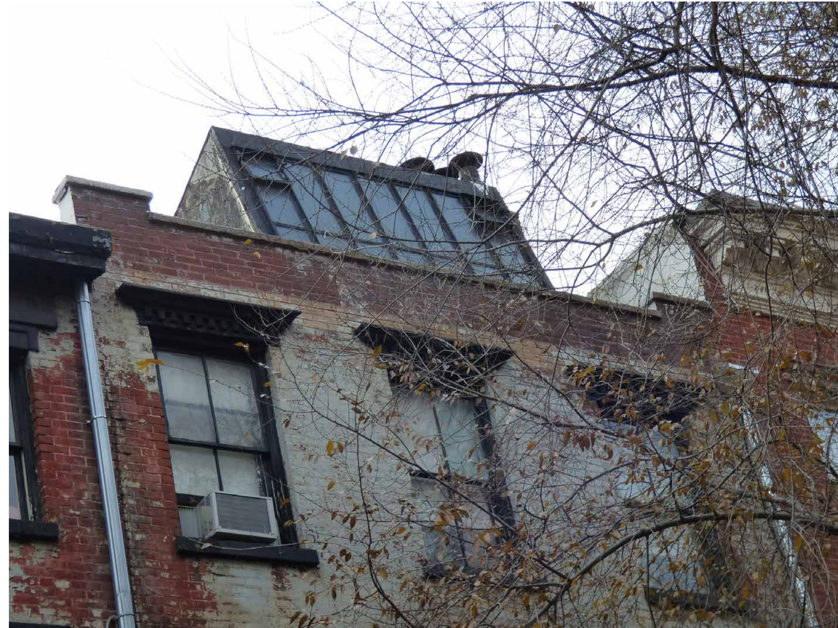
STUDIO WINDOW ADDITION (1930), CORNICE REMOVAL AND INCREASED WINDOW HEIGHT AT TOP FLOOR (1930?). NON-MATCHING BRICK ABOVE TOP-FLOOR WINDOW LINTELS.
