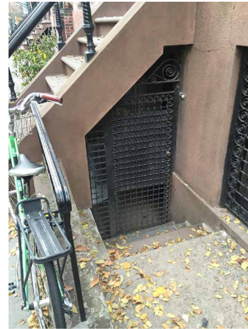
EXISTING GARDEN LEVEL ENTRY GRATE AT 246 WEST 11TH STREET TO BE REPLACED
