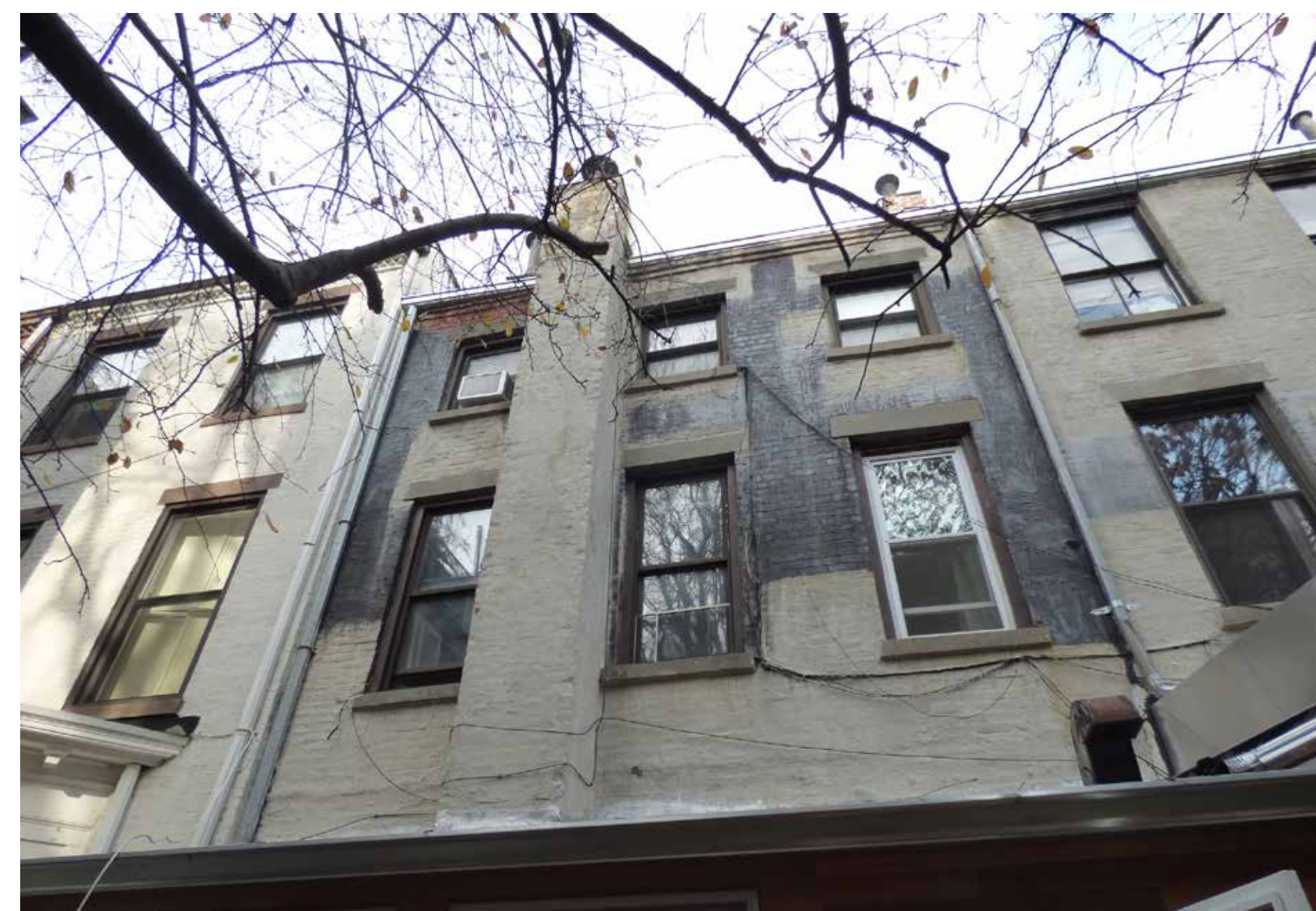
REAR ELEVATION. NON-ORIGINAL CHIMNEY, ADDITION OF MASTIC COATING AND PAINT. REPLACEMENT WINDOWS WITH CONCRETE SILLS AND LINTELS.
