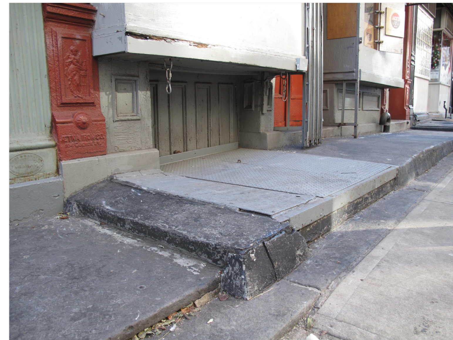
2 PHOTO - VAULT ACCESS HATCH
