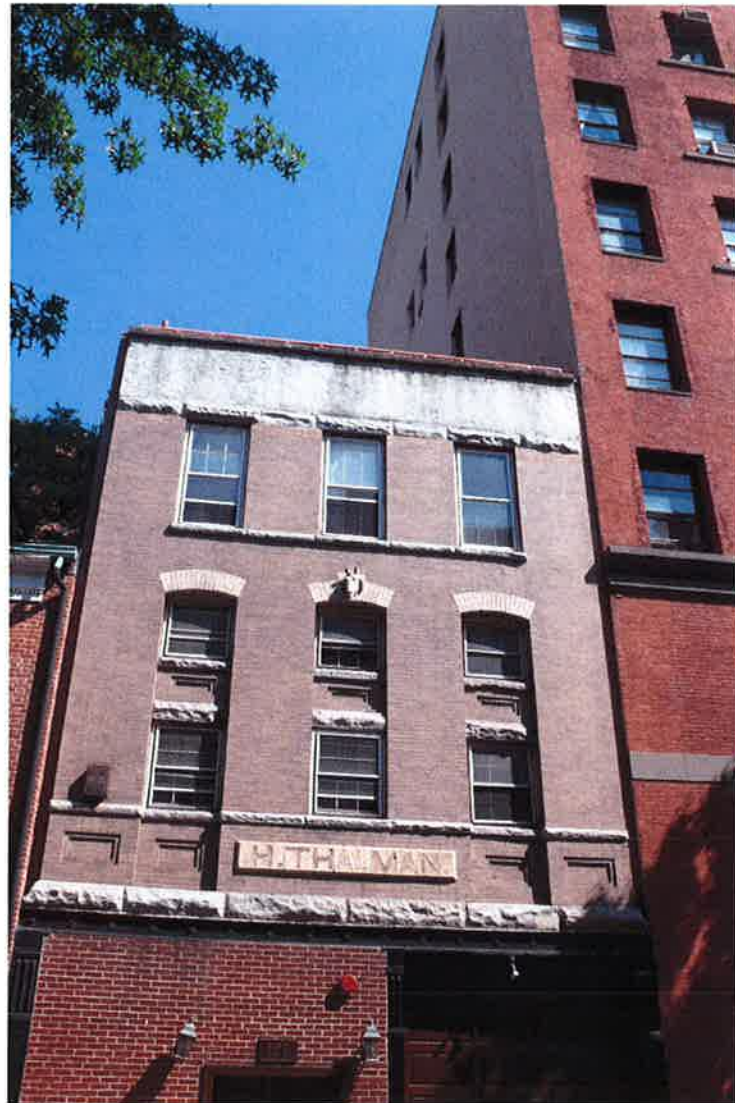
MATERIAL EXISTING BRICK MASONRY TO BE REFURBISHED AS REQUIRED LOCATION FRONT (SOUTH) ELEVATION ITEM FRONT FACADE
