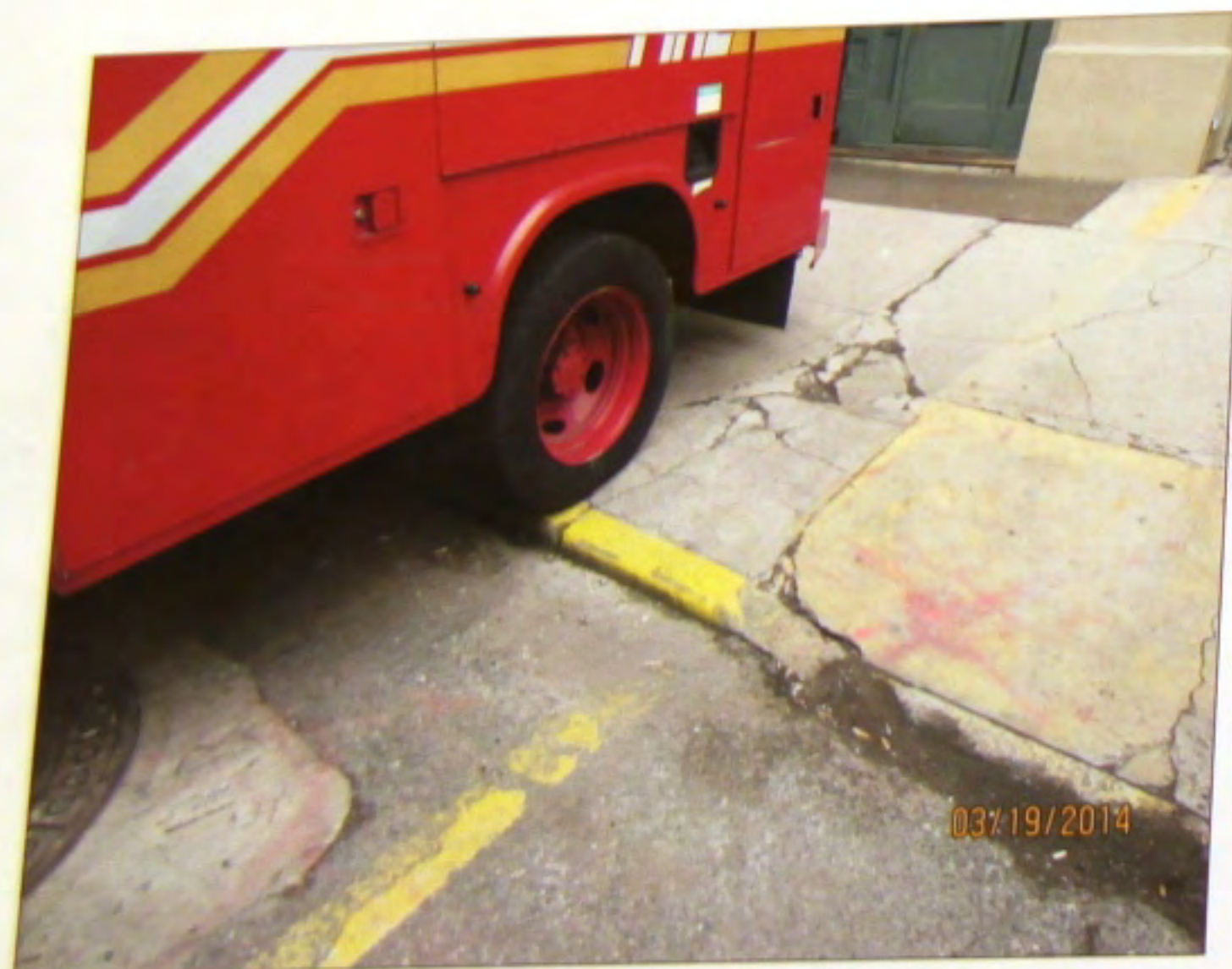
PHOTO 4 4 SCALE: NTS S-102 CURB & SIDEWALK AT WEST SIDE OF RAMP
