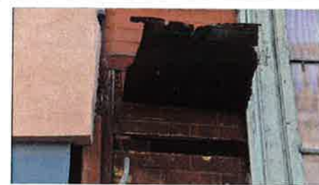
9 PHOTO OF EXISTING SIDING NTS
