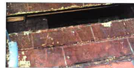
10 PHOTO OF EXISTING SIDING NTS
