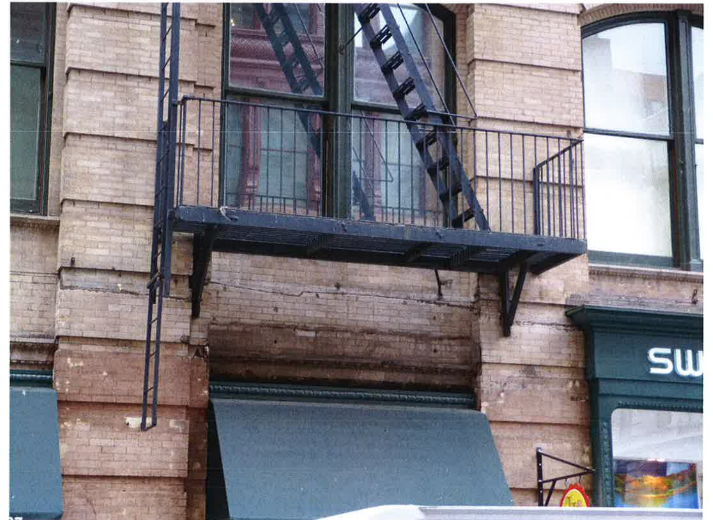
Deterioration Beneath Fire Escape and Above Storefront on Bleeker Street
