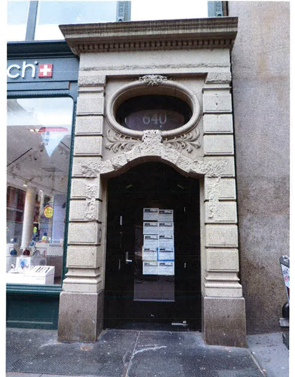
Painted Limestone and Missing Ornament at Entry on Broadway
