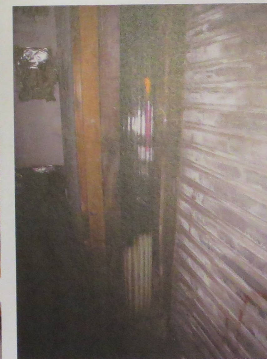
CONCEALED CAST-IRON COLUMN (BOTTOM)
