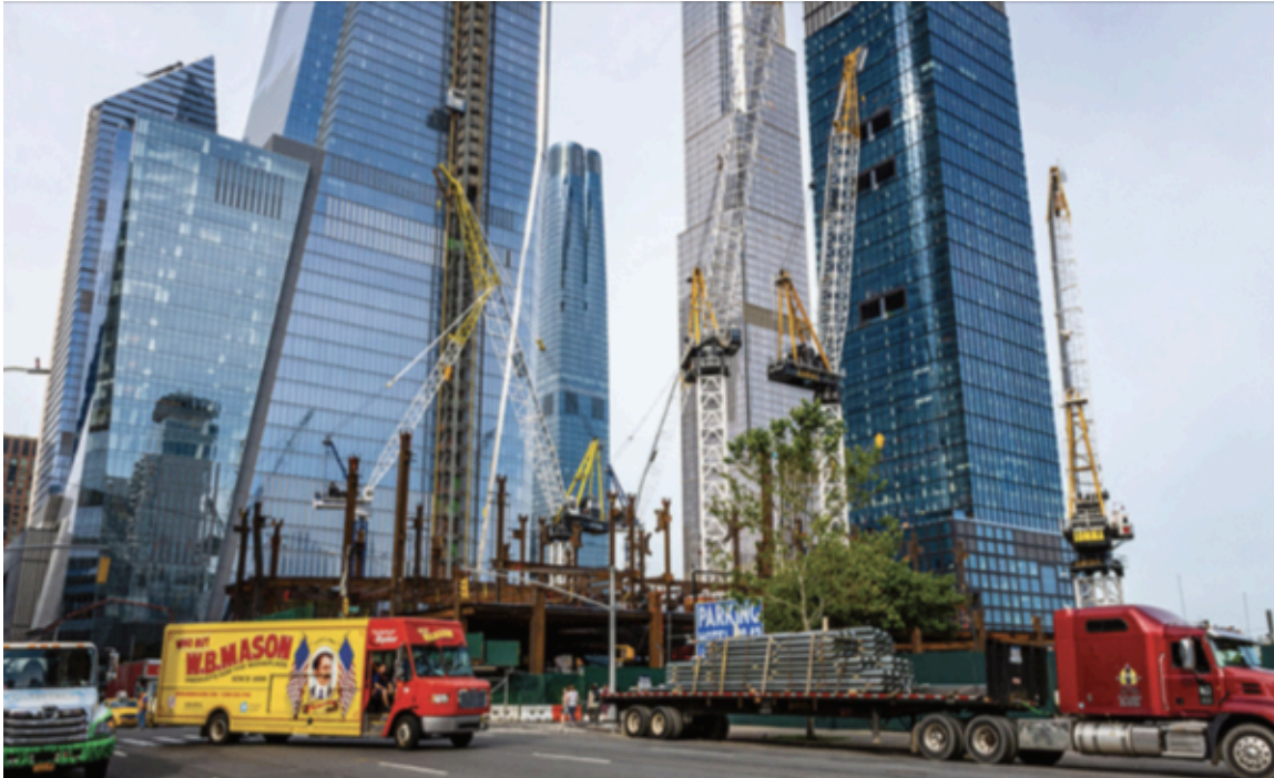
Manhattan Hudson Yards construction sites next to skyscrapers. Photo courtesy of Village Preservation.
