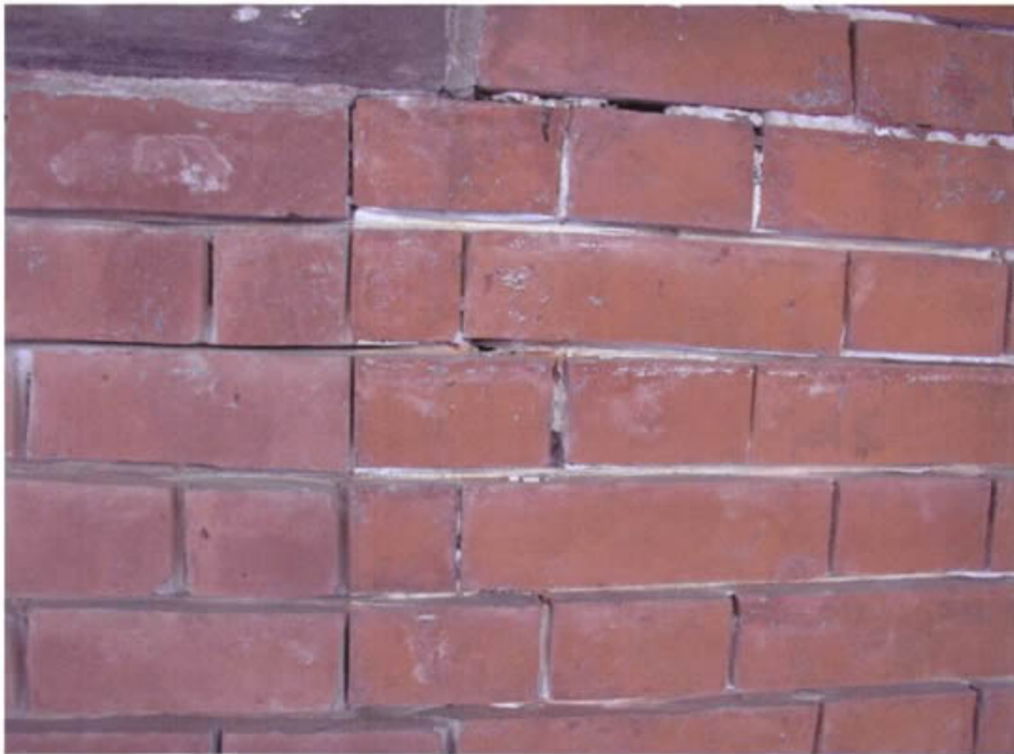
Photo 2: Poorly executed cutting of mortar joints is not only unsightly, but will affect the longevity of historic bricks. Note the unevenness of the grinder cuts. Joints should have been hand-cut if mortar removal was necessary.
